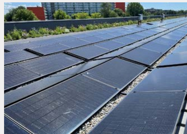
Full utilisation of flat roofs for PV panels
